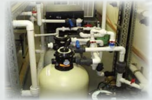
Water filtration equipment.
